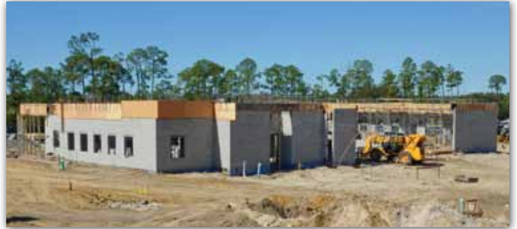
Construction is under way for two new buildings on the Collier Campus, including the Student Services Building.
