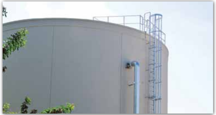
The new Thermal Energy Storage System is now fully operational on the Collier Campus.
